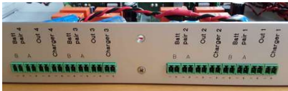
Figure 3: Battery, output and charger terminal block connectors in rear panel. This model has place for four battery pairs.
