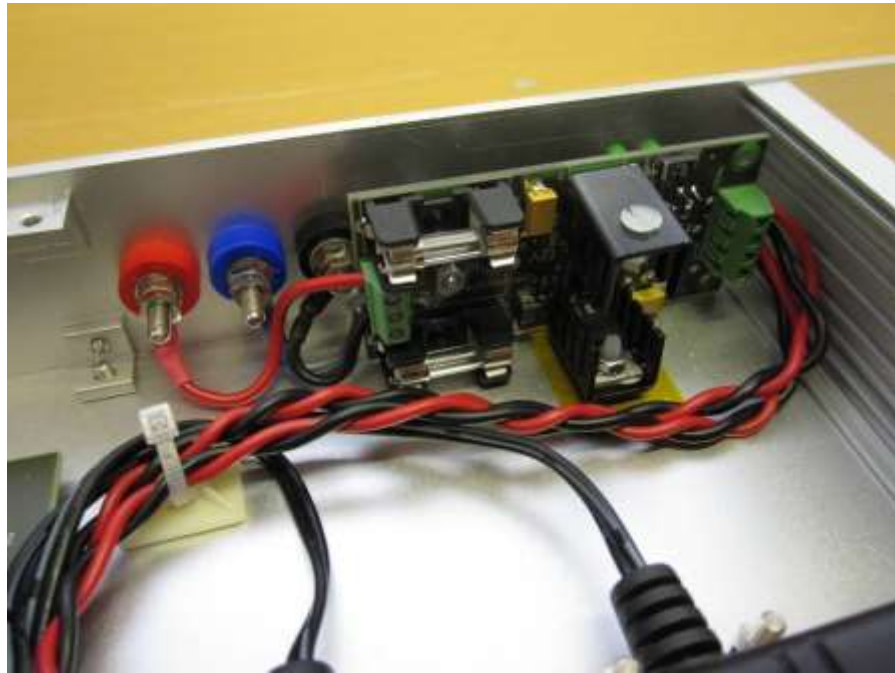
Figure 6: Voltage regulator unit with fuses. If there is no voltage at the regulator output but the leds are on (and regulator switch is on), check the fuses.
