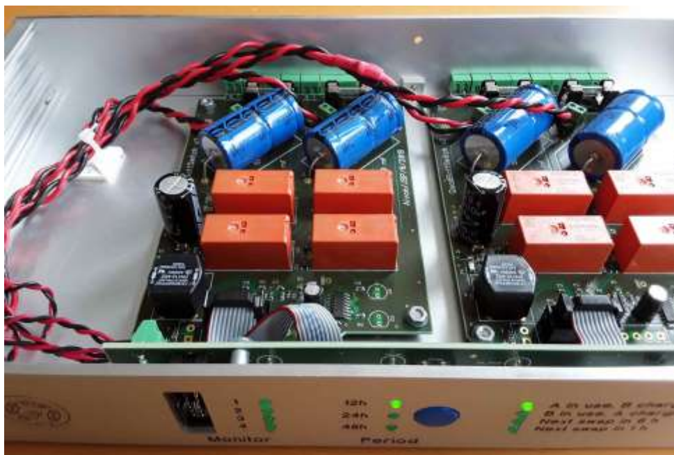
Figure 1: Two identical boards for 2 battery pairs including relays and storage capacitor. Glass fuses next to rear panel.
