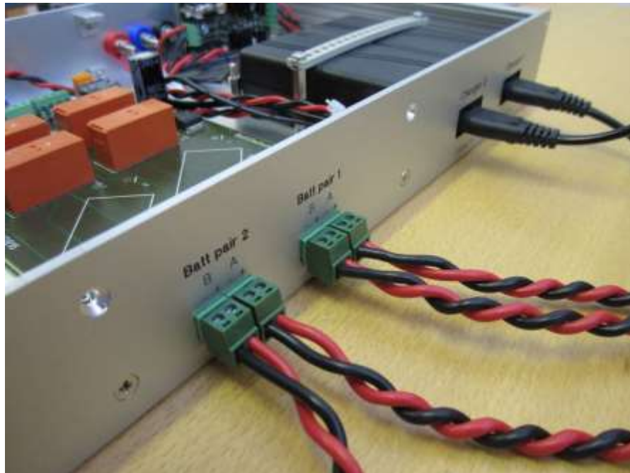
Figure 8: Connections for batteries and charger power cords.
